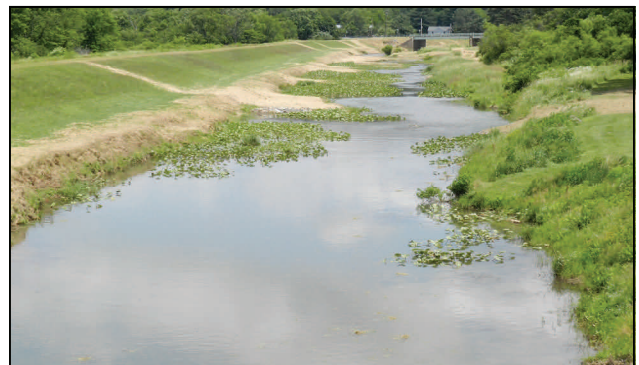
After: Phase III installation of habitat devices and stream bank stabilization have been completed.
